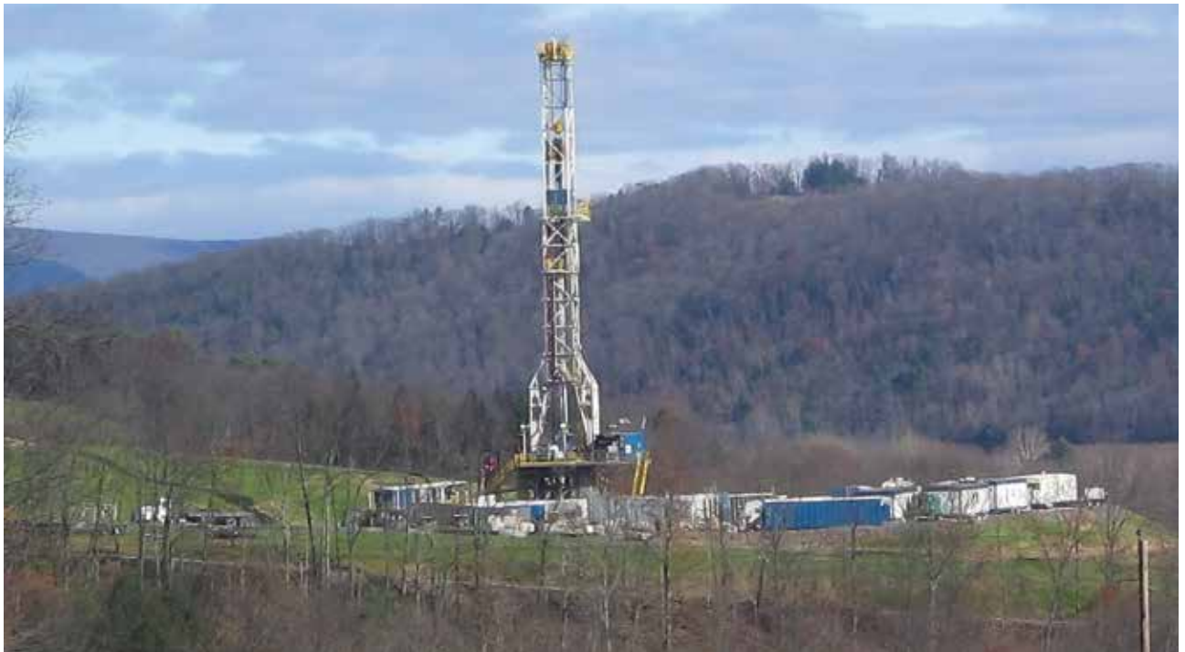
Figure 2.2: Tower for drilling horizontally into the Marcellus Shale Formation for natural gas in Lycoming County, Pennsylvania, USA
